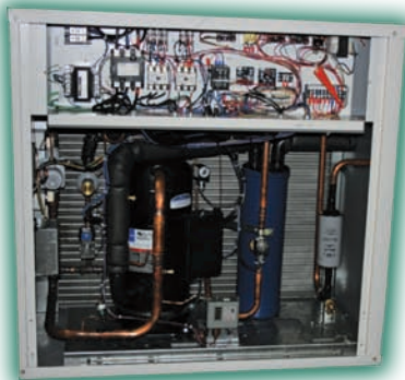
Interior of 100% Outside Air Unit (RCA Model)
